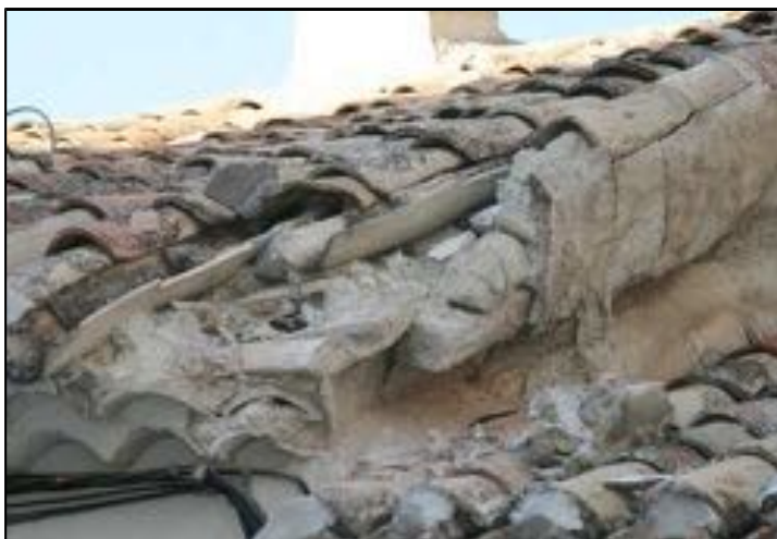
Figure 14. Image of start of roof deterioration in the old town (own photo)
