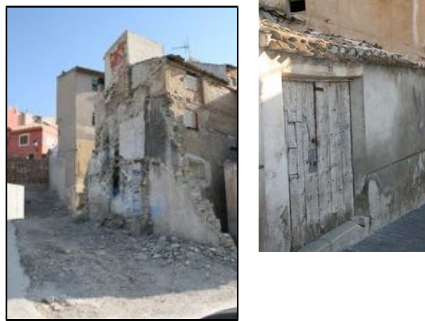
Figure 7. Image of dilapidated edification (own photo)
